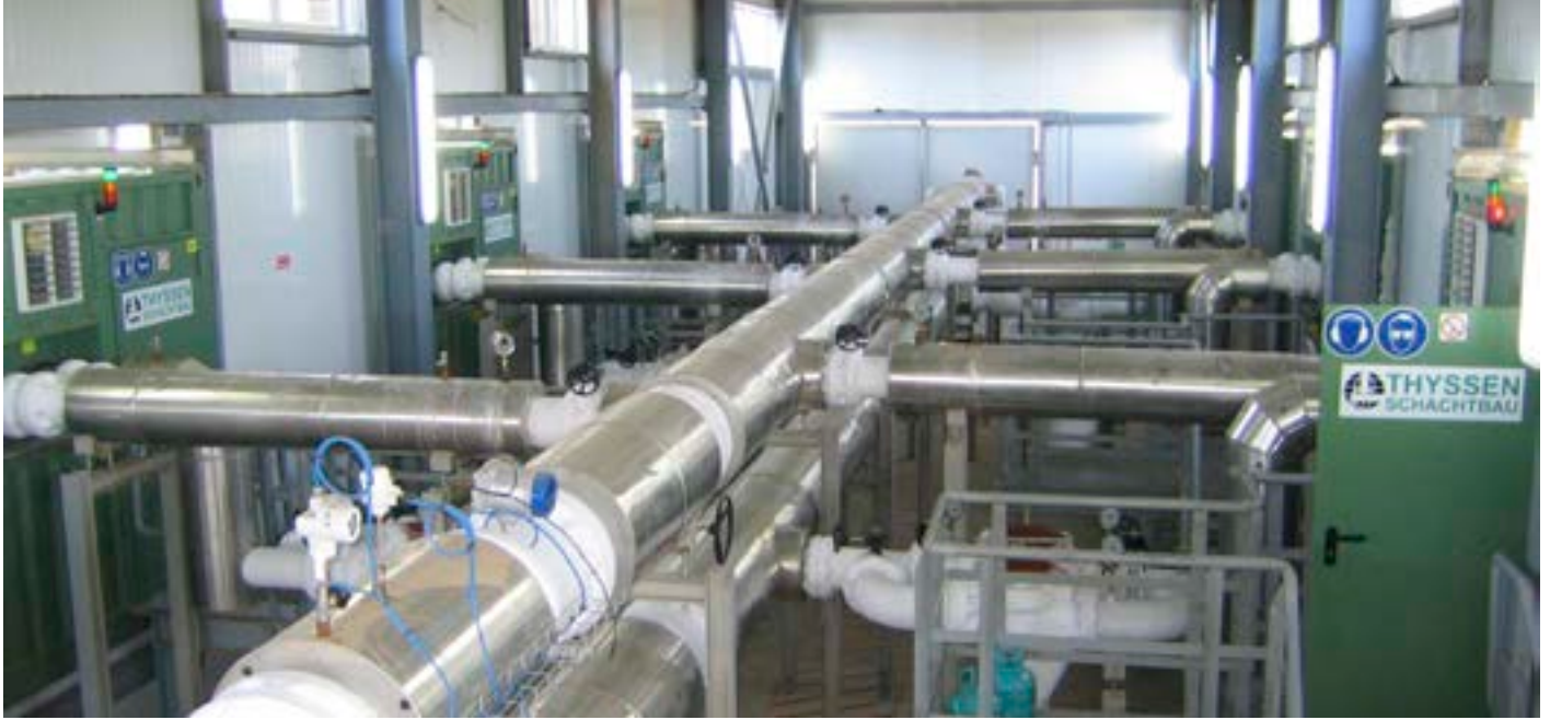
Massive pipelines branch off from the pump house to the individual containers where the freezing systems are located.
